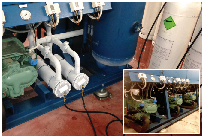
A medium temperature (MT) refrigeration rack from a R-404A/CO 2 hybrid system in a supermarket in Milan was converted to Opteon™ XP40 (R-449A).
